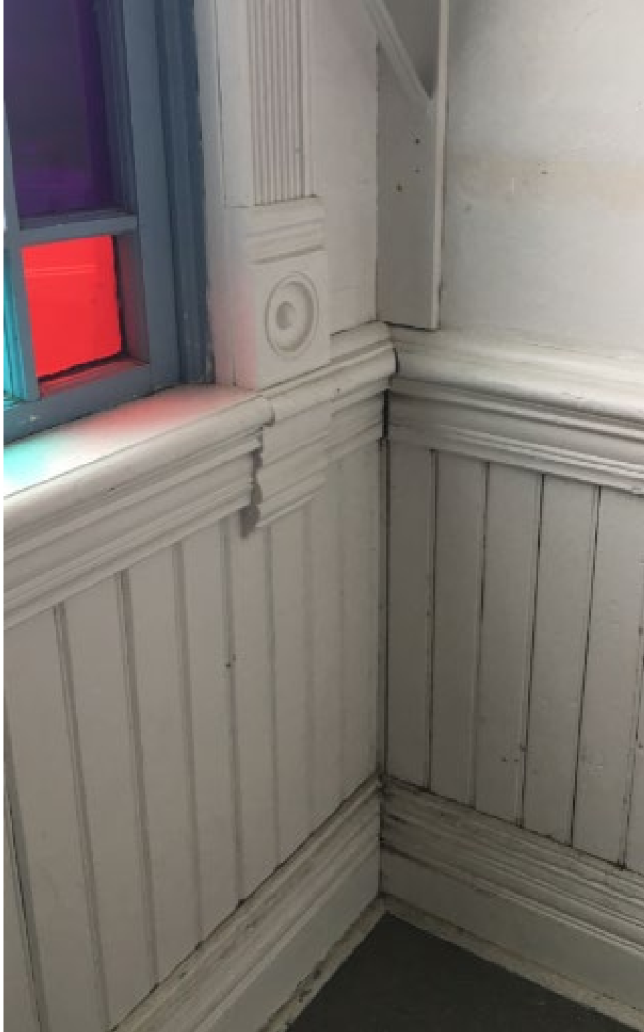
1892 decorative interior mouldings include 9 ½" tall base, 30" tongue and groove wainscoting below 7" chair rail, window apron, rosette plinth blocks and 5 ½" wide fluted casing.
