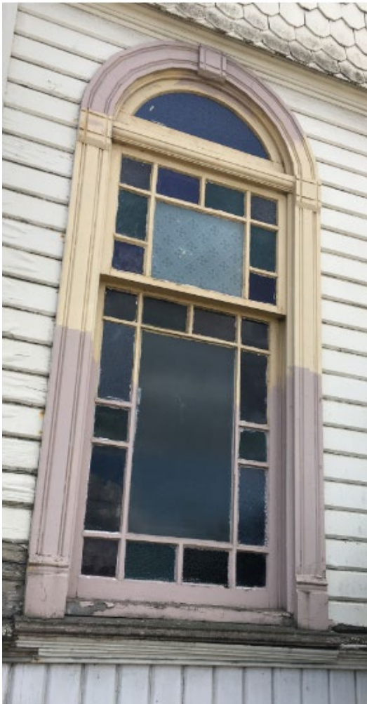
Colored glass, true divided lite double hung window with half round transome window, north front
