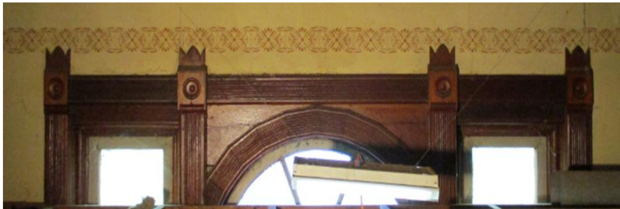
Unstained interior fluted window casing for ganged window unit, on north front of church. Top half of wheel window with arched fluted casing visible. Decorative crowns top the rosette style corner blocks.
