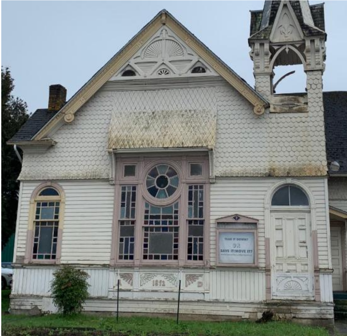
Church front, north side along Santiam Road showing central wheel window and ganged true divided light windows. Original Entry on right side of photograph.
